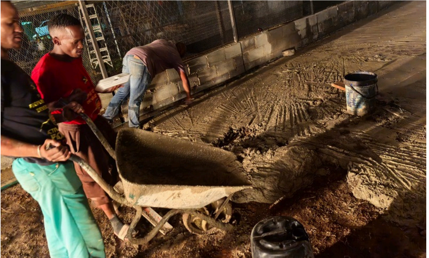
Nutrition boost: Laying the foundation of the chicken coop after completing the enclosure, after which the cages for the layers were assembled. Ganspan, Northern Cape.
